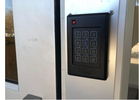
Safety & Security- Access Controls
